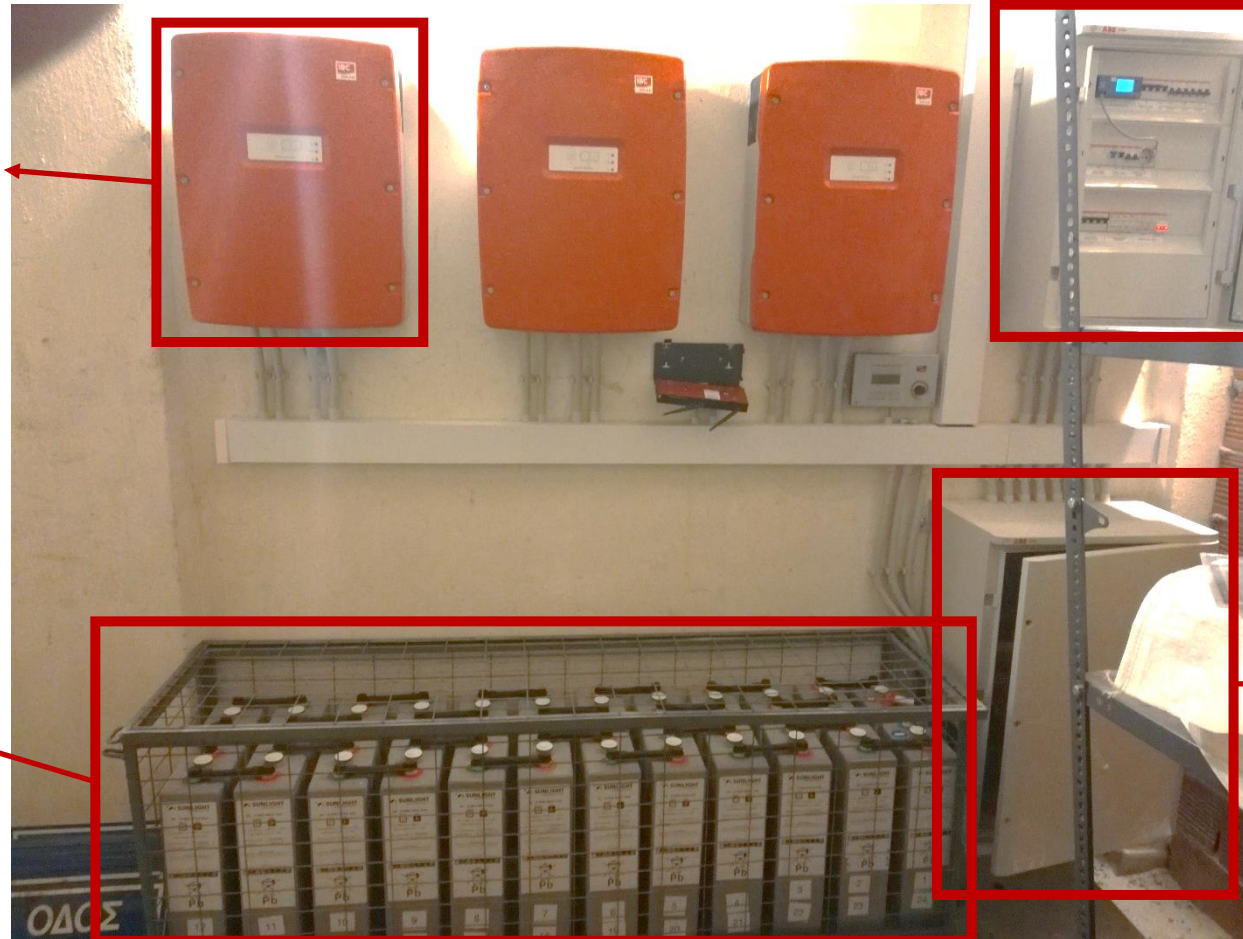
1-phase Battery converter
